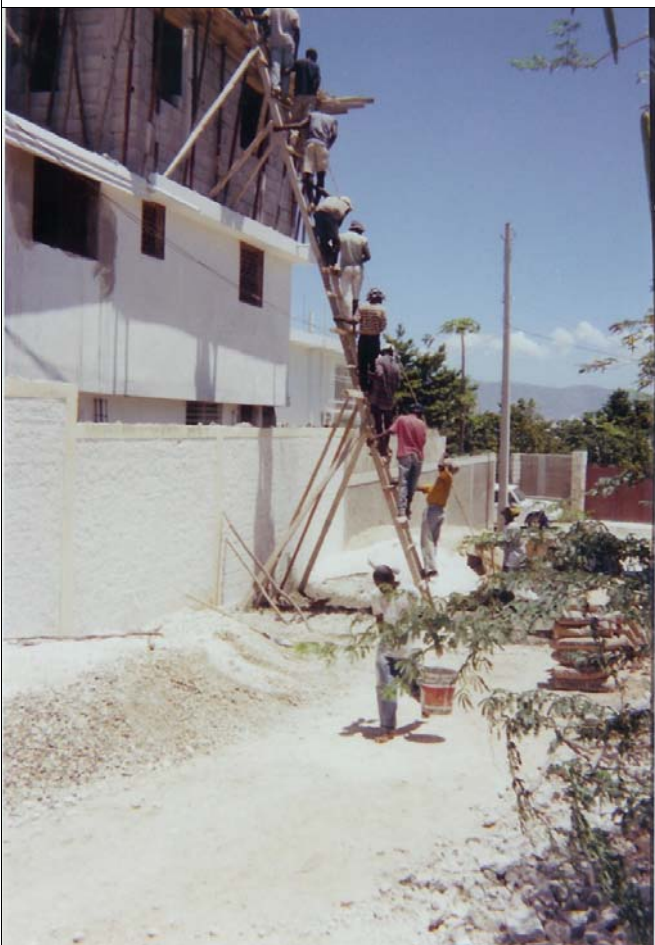
Haitian workers haul concrete up a ladder to the roof of our new Mercy Clinic building, bucket-by-bucket...
